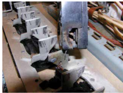
FPRF, Service Panel from Sample Home, Arcing Damage
