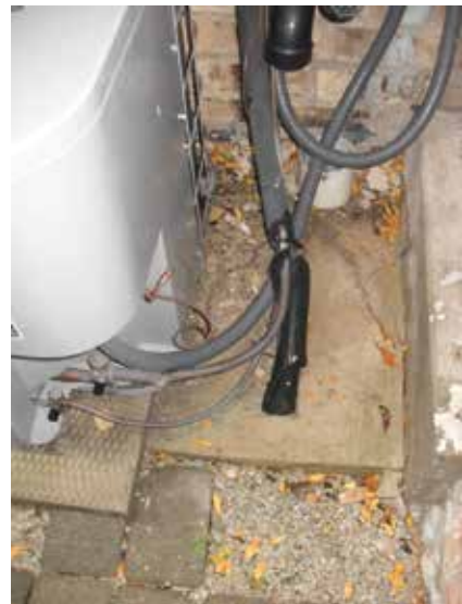
Connection near the condenser is a common area for leaks
