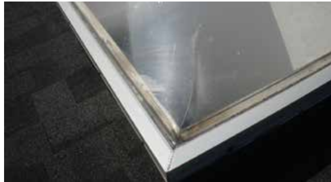
Look carefully – cracks are easy to miss
