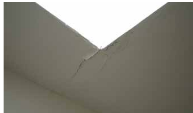
Look from the inside for damage and leaks
