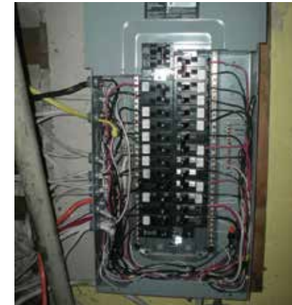
There is no ground wire coming out of the main disconnect part of this panel
