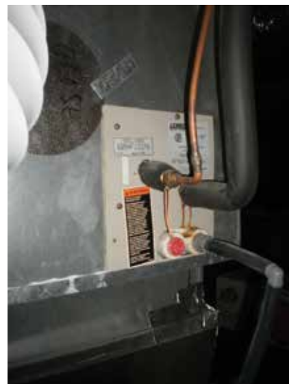
Stains below the suction line indicate leaking
