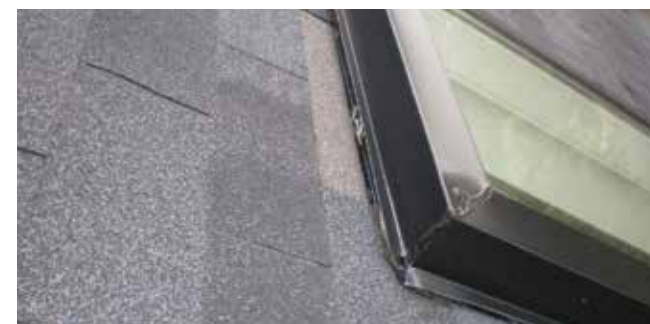
Roofing material missing
