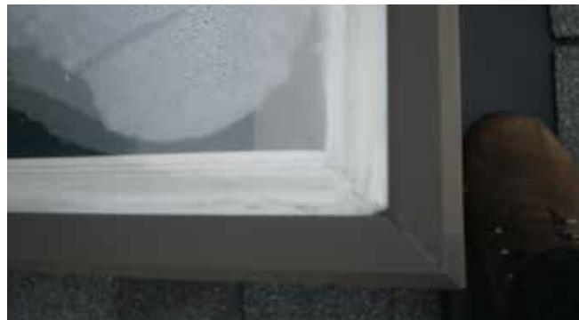
Sealed units should not have condensation
