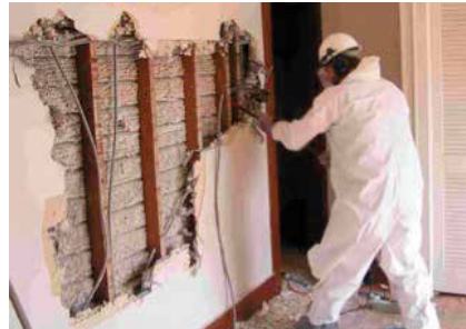
FPRF, Recovering Wiring from Test Home in Chicago, IL.
