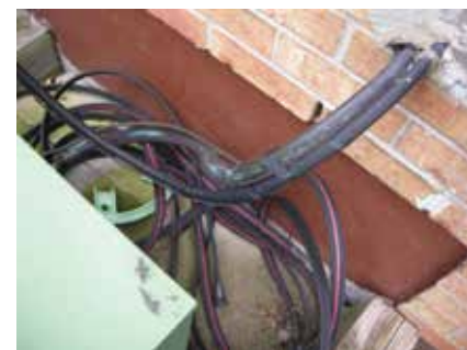
Suction line is missing most of its insulation
