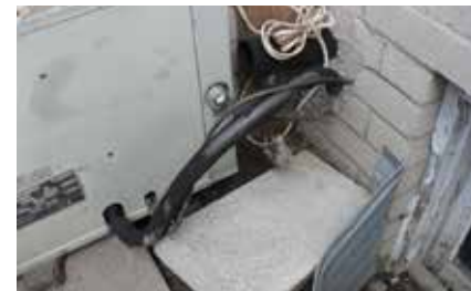
Damaged insulation due to vermin activity
