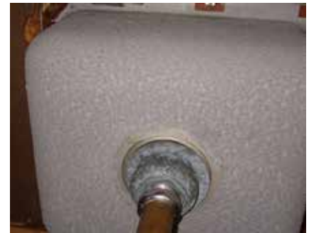
Photo: Asbestos-containing insulation on the underside of a metal sink is added to prevent condensation, but it can become brittle over time. Courtesy Asbestorama
