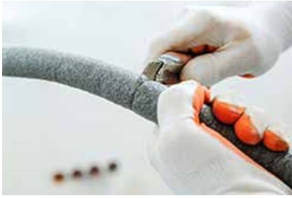
Photo: Asbestos insulation around pipes is not uncommon and cutting the insulation could disperse asbestos fibers.
