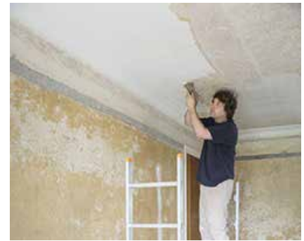
Photo: Scraping popcorn ceiling containing asbestos can be hazardous without proper masks and ventilation.
