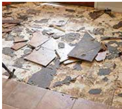
Photo: Loose vinyl tiles with exposed asbestos-containing adhesive.
