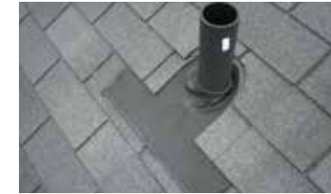
A poorly installed flashing may leak and will reduce its life expectancy.
