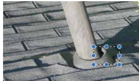
The flashing boot is recessed and will hold water.
