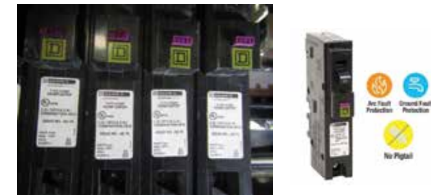
Dual Function GFCI/AFCI Breakers Found Recently at a New Build Home – This is a No Pigtail Style Note: Square D Dual Function Breaker Reset Button Is Color Coded Purple – Right Image by Square D
