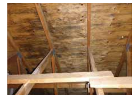
Mold on sheathing suggests issues with attic moisture
