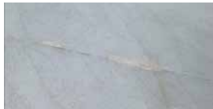
Poorly sealed synthetic stucco (EIFS) can have serious implications
