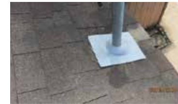
Improper installation - flange is on top of the shingles.
