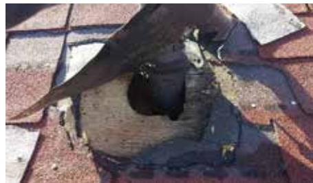
Stack flashing and shingles damaged by vermin
