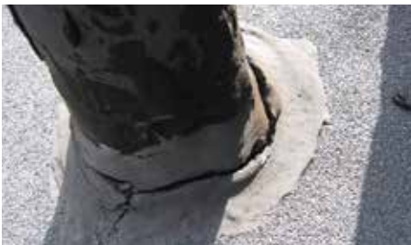
Roofing cement was used as the flashing material - a very poor approach
