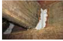
Crawlspace: Hangers – Only 5-6 Years Old and Again – We Have Problems
