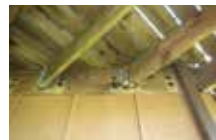
Elevated Deck, Coastal Environment, Less Than 7 Years Old. Note Corroded Bolts, Right Hanger is Almost Completely Rusted Through
