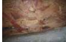
Crawlspace: Note Black Stains At Shear Nails In What Appears To Be A Dry Environment – Sick Nail Syndrome?
