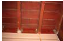
Exterior Stair Landing: 7-9 Years Old – Note Rust Dripping From Hanger
