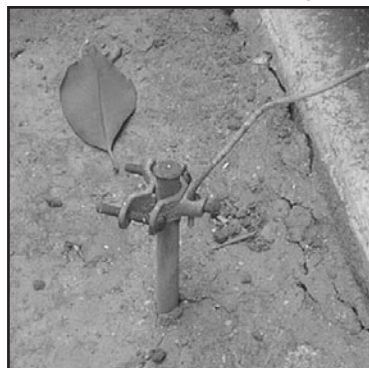
Figure 8 — The clamp is oriented correctly, but the conductor is unprotected.
